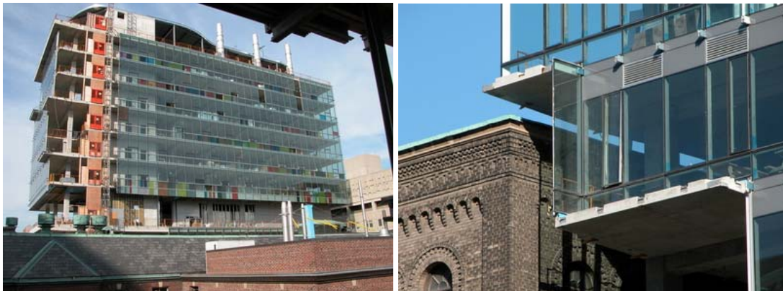
Figure 12: Innovation and Design Process: Centre for Cellular and Biomolecular Research, University of Toronto, Benisch and Benisch. Double skin façade construction in progress. The building also uses innovative planning to separate less climate controlled corridor spaces from highly controlled laboratories. Two storey planted atriums will be located at the corners of the south face of the building.
