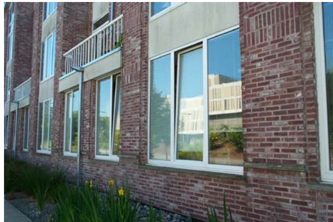
Figure 9: C.K. Choi Institute for Asian Studies, UBC, Matsuaki Wright Architects Indoor Environmental Quality: Ventilation Effectiveness + Control of Perimeter systems
