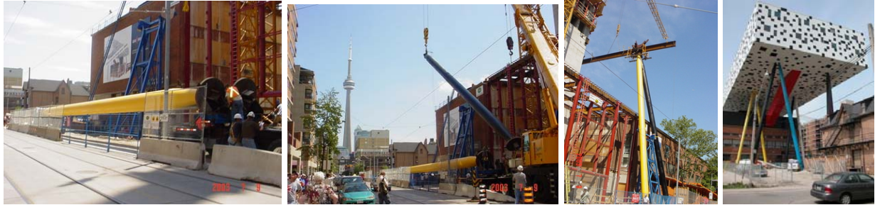
Figures: Erection sequence for HSS legs on OCAD project. Photos: PCL Construction.
