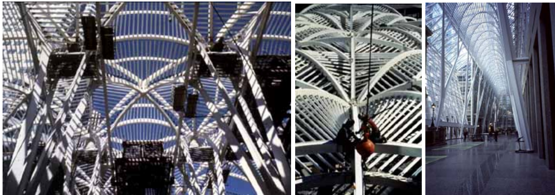
Figures: BCE Place, construction and finished images. Excerpted from SSEF Case Studies CD-ROM Volume 1.
