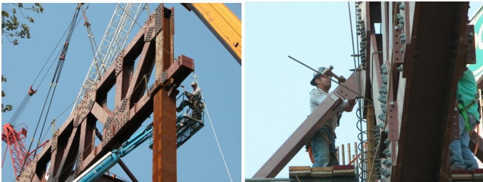
Figures: Leslie Dan School of Pharmacy, University of Toronto, Norman Foster – erection of a 50 tonne steel truss at the fifth floor level.
