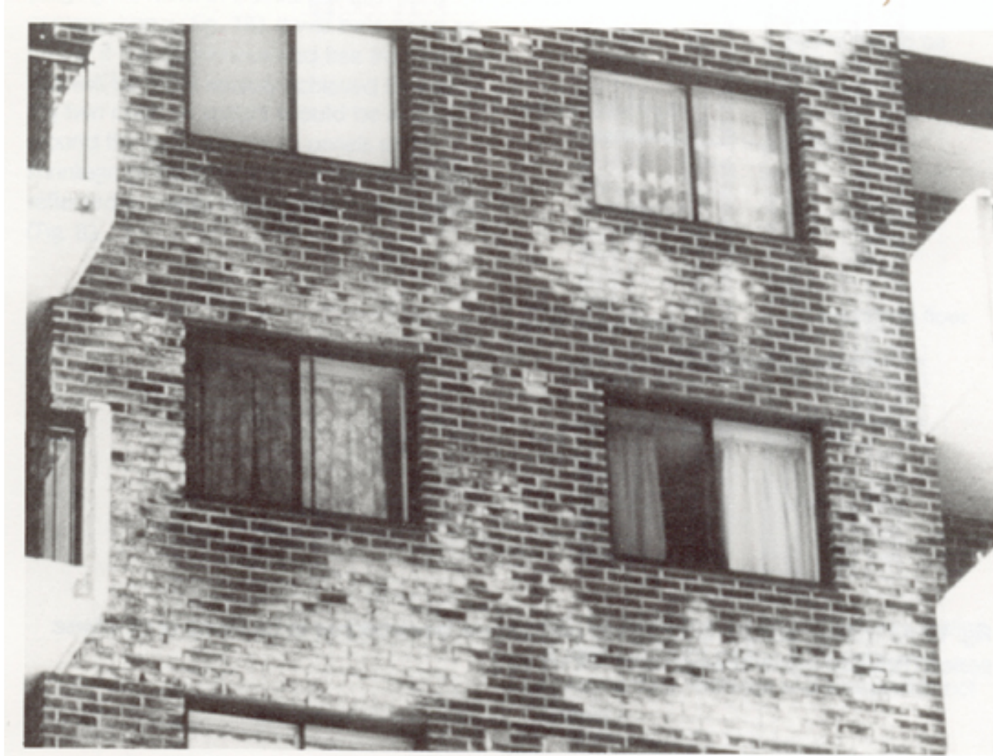
Fig. 16 An example of extensive wetness and efflorescence
