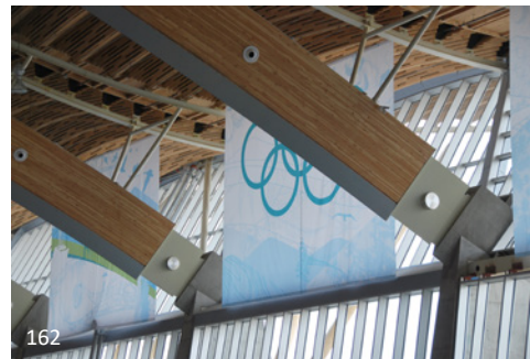
162 The large arches over the Richmond Speed Skating Oval are fabricated from a combination of steel and wood, with the majority of the steel hidden beneath the wood cladding of the arches.
