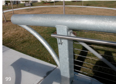
99 Seal welds have been used to connect the various components of this exterior galvanized steel feature railing. There is a large opening at the base of the square HSS post to allow any water that may enter the railing an opportunity to drain.
