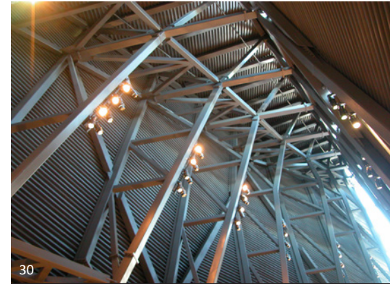
The Canadian War Museum in Ottawa uses AESS to create a highly articulated and rugged expression of the steel in Regeneration Hall. In this instance a combination of welded connections and exposed plate-to-plate moment connections at the connection points between square HSS sections is the feature of the appearance. Due to the irregularity of the structure, tight tolerances are required. The profiled decking is also left exposed to view.
