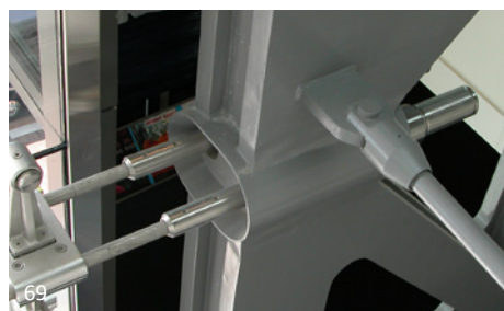
Fig. 4.2B It is easy to see that this detail relies on a high level of finishing – including grinding and contouring of the welds to achieve its form, fit and finish.
