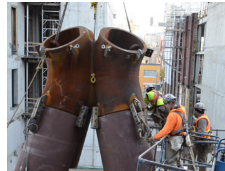
134 A large cast node was used to resolve the geometry of this large tubular support structure.
