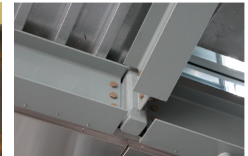
64 Fig. 3.5B This exposed bolted connection is tightly designed and demonstrates uniformity in the joint gaps.
