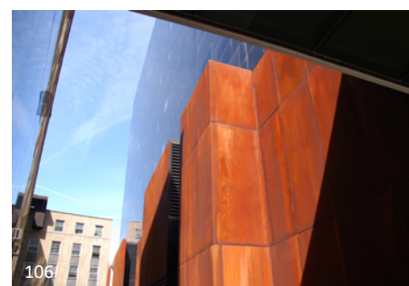
106 This wall is made from weathering steel. The final colour of the steel will be slightly darker than what is pictured here. The material must go through a number of wetting and drying cycles for the coating to cure. It is not possible to select or carefully predict its final hue.
