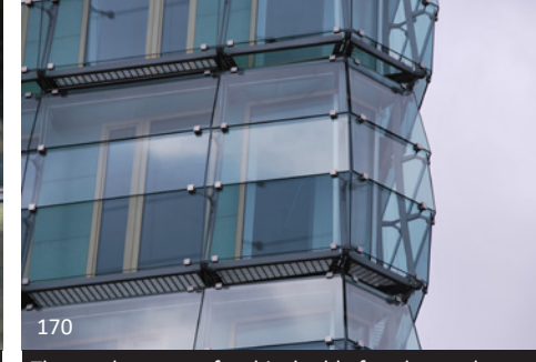
170 The steel supports for this double façade envelope use a system of clips to support the extra layer of glass. This alleviates issues of drilling of the glass and allows for better accommodation of differential movement between the systems.
