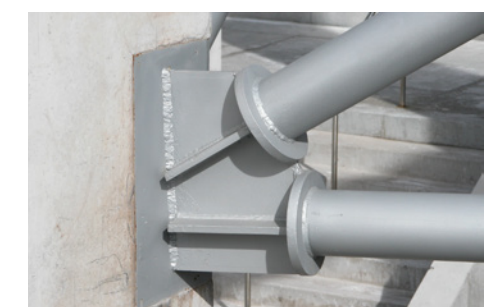
66 Fig. 3.6B This design used all-welded connections, even for this anchoring detail of the truss to the base plate. Bolted connections were not desired.
