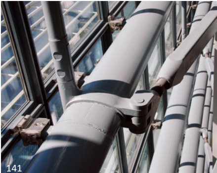
141 Elliptical tubes are a new product that is seeing increasing use. These tubes are used to support a high curtain wall in an airport. The weld seam is located on the top of the member as the predominant viewing angle is from below.
