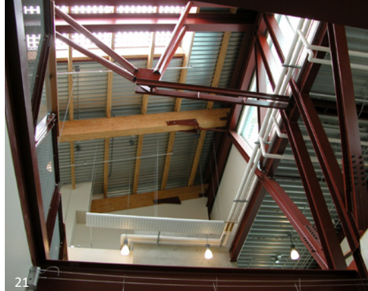
National Works, Vancouver B.C.: The project uses a more articulated steel design, predominantly with W-sections. Much of the structure is located at ceiling height, so at a distance for viewing and therefore allowing for a lower level of detailing and fine finish. This structure interacts with wood, which will change aspects of its detailing and coordination during erection.
