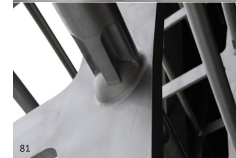
The Chinese National Theatre uses large plate steel members to create its trusses. These in turn are braced by solid rods that use a half-sphere to manipulate the curve of the connection. The form, fit and finish on the project are very high. This was undoubtedly the result of significant coordination and close supervision of the work.
