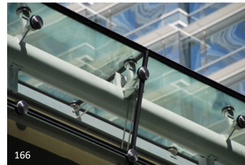
166 Spider connectors are used to connect this mullionless glass to a tubular steel frame at the top of the expanse of window of this Las Vegas Hotel lobby. The coordination for this detail is extremely tight, with little room for discrepancy given the proximity of the steel tube to the inside face of the glass.
