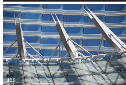
165 A suite of articulated steel arms cantilevers out over a hotel drop-off area. Diagonal rods with stainless connectors support the glazed roof.
