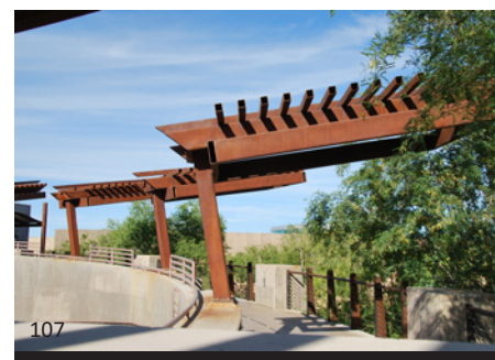
107 Care must be taken in detailing weathering steel to avoid having the natural oxidizing process create stains on the surfaces below the material.
