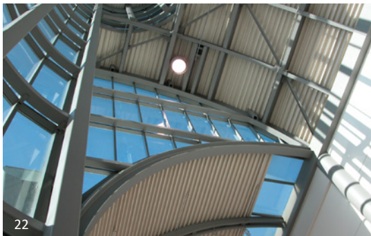
Direct Energy Centre, Toronto, ON: The project makes use of relatively standard steel sections, but the design and fabrication employ a higher standard in terms of arrangement and detailing. There is some section bending required which increases fabrication costs and can impact detailing. Much of the structure is still located in excess of 6 metres above view.
