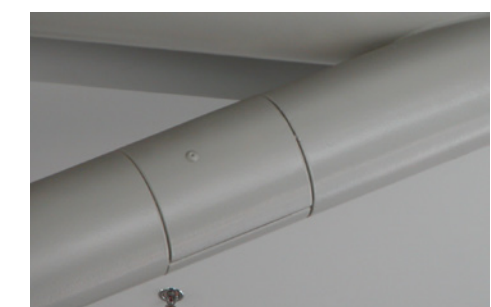
65 Fig. 3.6A Pictured is a cover plate over a hidden bolted connection. The appearance of a completely welded structure is kept, but erection simplified.
