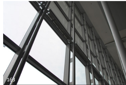
163 The AESS system illustrated here uses a specialized vertical truss-like column formed from round HSS sections and plates, with holes cut into the plates to lighten the appearance of the system, to act as the lateral wind load support for this very tall expanse of glass at Pearson Airport. The thin profile of the steel appears as a simple extension of the curtain wall.
