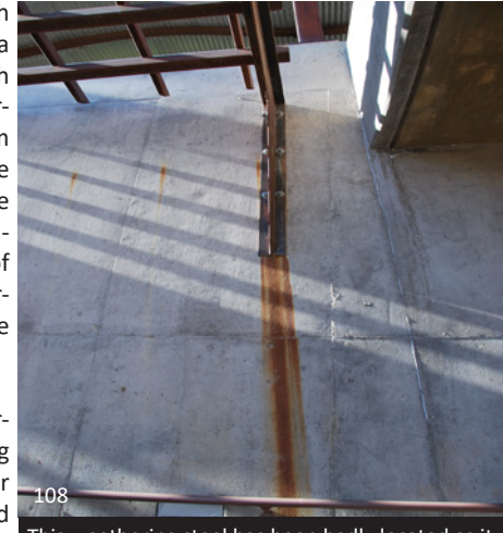
108 This weathering steel has been badly located as it is staining the concrete wall below.
