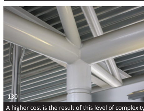
129 It was important for the form, fit and finish in this building to have a seamless transition between these two HSS members, so a welded connection was used. All evidence of the joining of the two members was concealed.
