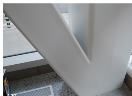
128 The large HSS members used on this bridge have helical welds. Although unusual in appearance, they were aesthetically worked into the design.
