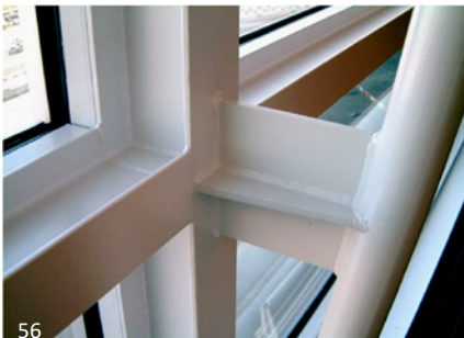
56 Fig. 2.4B Welds are plainly visible but of good, uniform quality so complimentary to the structure.
