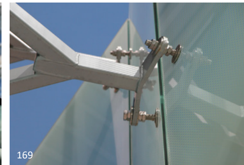
169 Alignment issues between the glass and steel support frame are taken care of by levelling mechanisms that are part of the glass connection system. These are located on the rear of the canopy and are not visible from the front, allowing for clean lines and uniformity on the public side of the system.
