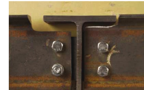
63 Fig. 3.5A Joint gap minimized. The gaps on the left are standard structural steel, and on the right sized for AESS. (Courtesy of AISC)
