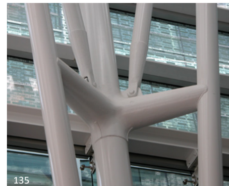
135 These cast connections made appropriate use of castings to resolve complex geometries cleanly.
