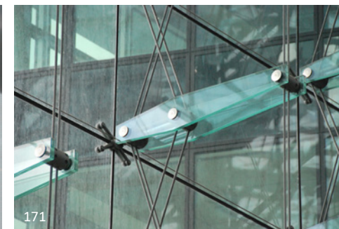
171 Stainless steel cables are used in conjunction with laminated structural glass and stainless spider connectors to support this large glazed façade at a Berlin rail station.
