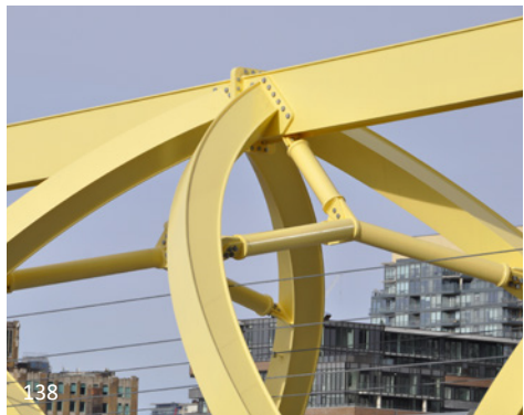
138 The curved box members of this pedestrian bridge were created via plate rolling. The use of plate provides crisp corners as suits AESS 4. The joining plates were inset to give a shadow line.
