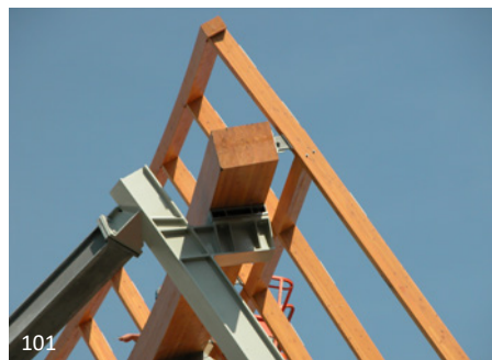
101 Here galvanized steel members are mixed with zinc painted grey steel. It was decided not to galvanize some of the members due to the chance of deformation in the hot zinc bath and potential stress release of the welds.
