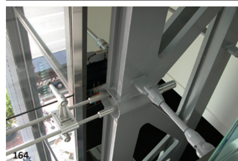
164 A highly articulated vertical truss at either end of a cable system is used to provide wind support for a large expanse of glass at the Newseum. Stainless steel clamps connect the spider connectors to the cables.
