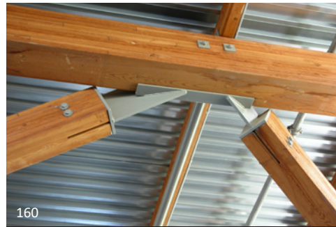
160 Steel connections are used to join this timber structure. It can be seen that the steel connection pieces are fitted with a plate that penetrates the end of the timber. Bolts through the assembly secure the plate to the timber. In this case the penetration slot is left exposed. These will often be filled or hidden to make the connections more mysterious.
