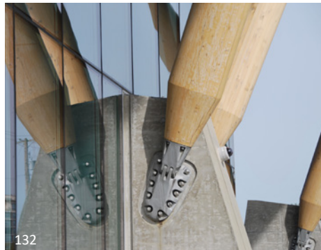
132 Custom castings are used to connect the timber columns to the concrete foundations.
