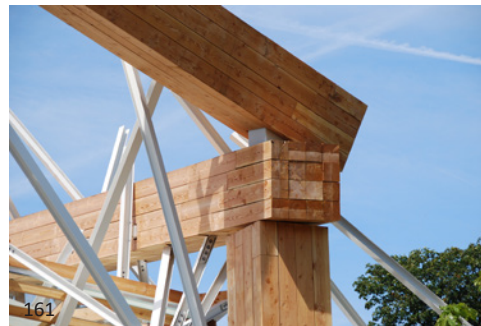
161 The heavy timber on this sculptural project is really “for show” as the main support system is all steel and the large square wood sections are used only to bulk out the form and provide a contrast with the steel used to support the glass.
