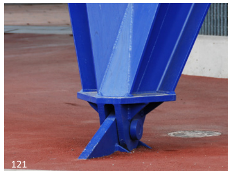
120 Welded connections have been used here in conjunction with the selection of W-members to create a very technical feel for the Works Yard.
