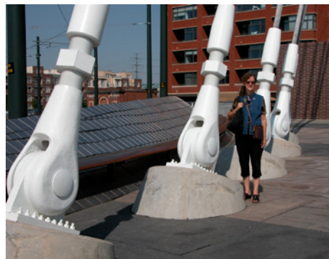
133 Castings used as tension anchors can vary greatly in size, from these pictured here to much smaller ones used to attach rods for stayed structures.
