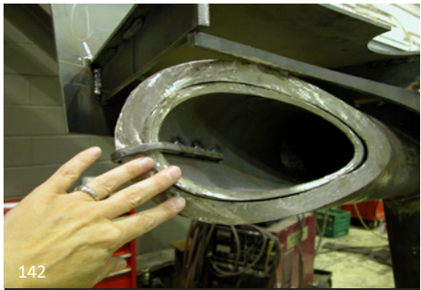
142 This curved section is distorted at its splice, making a smooth welded connection difficult to achieve.
