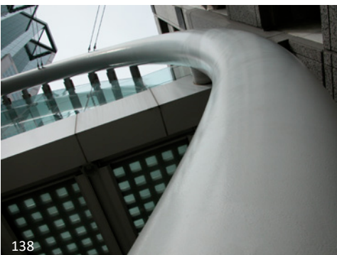
138 The high profile and very exposed nature of the round bent steel tubes that support this pedestrian bridge meant extra care in bending, splicing and erecting the structure.
