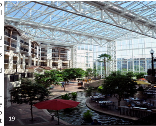
20 Gaylord Resort: The trusses that support the skylight are situated well above viewing level. They are fabricated from standard structural steel sections using primarily bolted connections. Aside from concern about the geometry and spacing there is not a lot of additional fabrication expense at this level.
