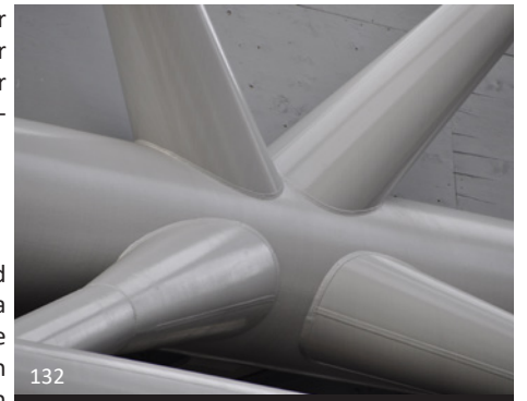
132 The welded seams on these custom conical elements have not been remediated.
