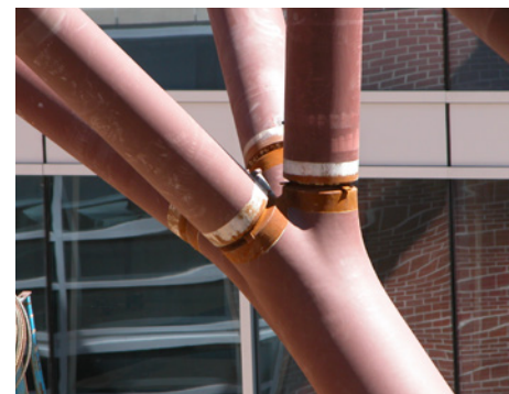
136 A large steel casting was used in this tree-like structure to join several mechanical pipe sections. The joints were filled and sanded to conceal them.
