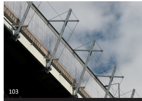
103 Galvanizing is a suitable finish for an exterior AESS structure that will be constantly subjected to weathering as in this expressive railing system.
